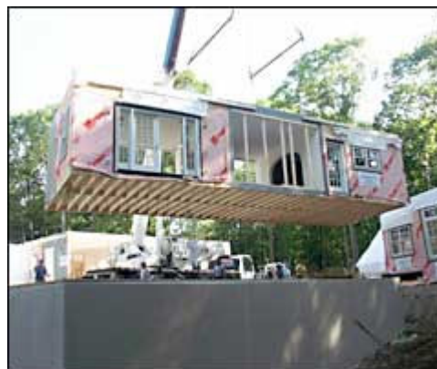
Direct from the factory. The first section of the Modular Mountain Retreat project house is lowered onto the foundation by a crane.
